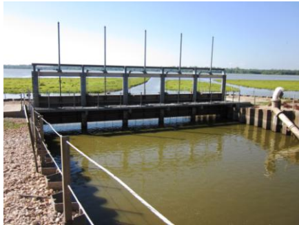
Lower Swan Lake pump intake
